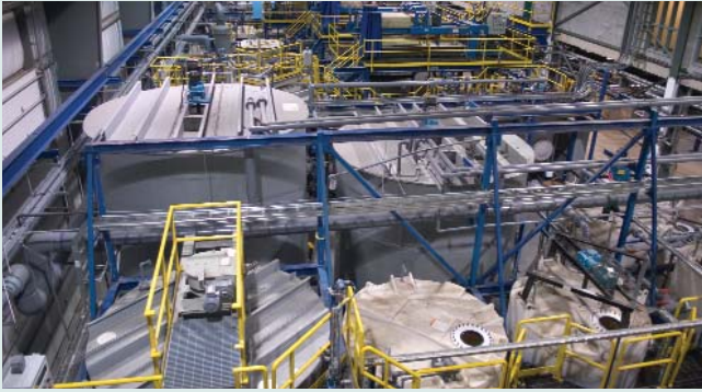
Demonstration Plant interior, Argentina
